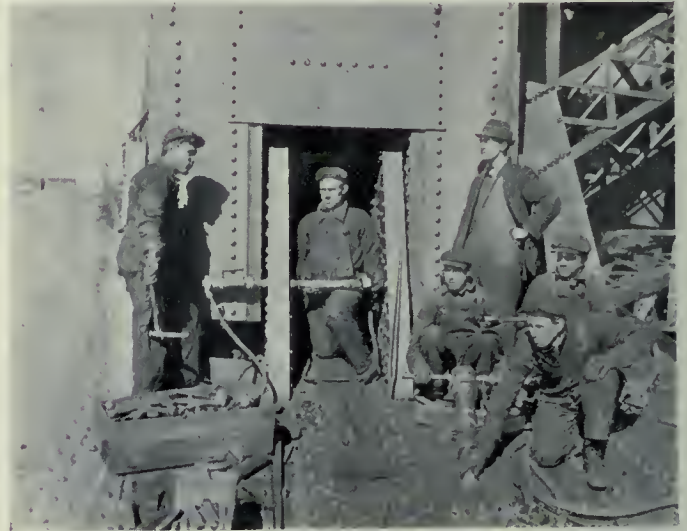
Fig. 3.—Panel point of bottom chord showing unusual dimensions of members—pneumatic buckler-up, hammer and rivet cutter at work.
